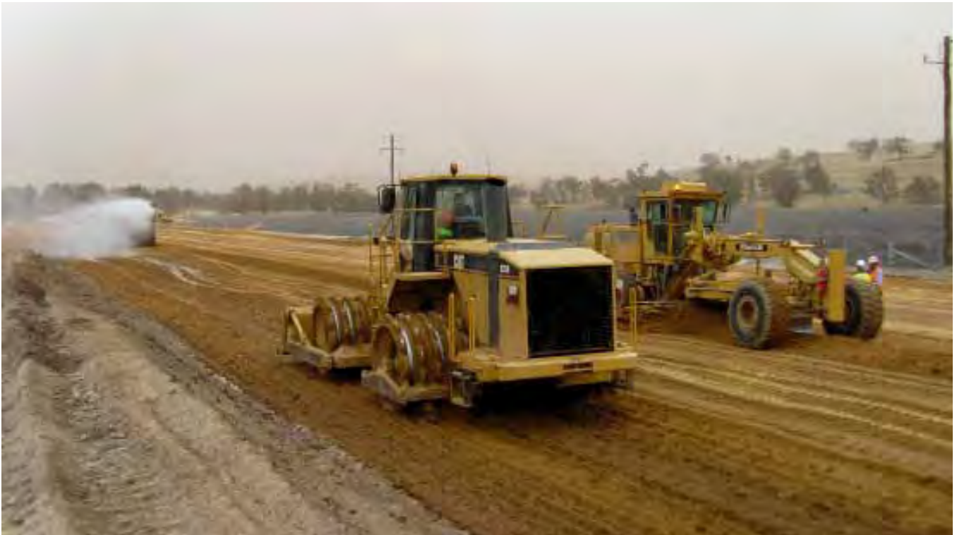
Water is an essential component during construction of road works, used in compaction of earthworks, dust suppression activities and revegetation of the construction site.
