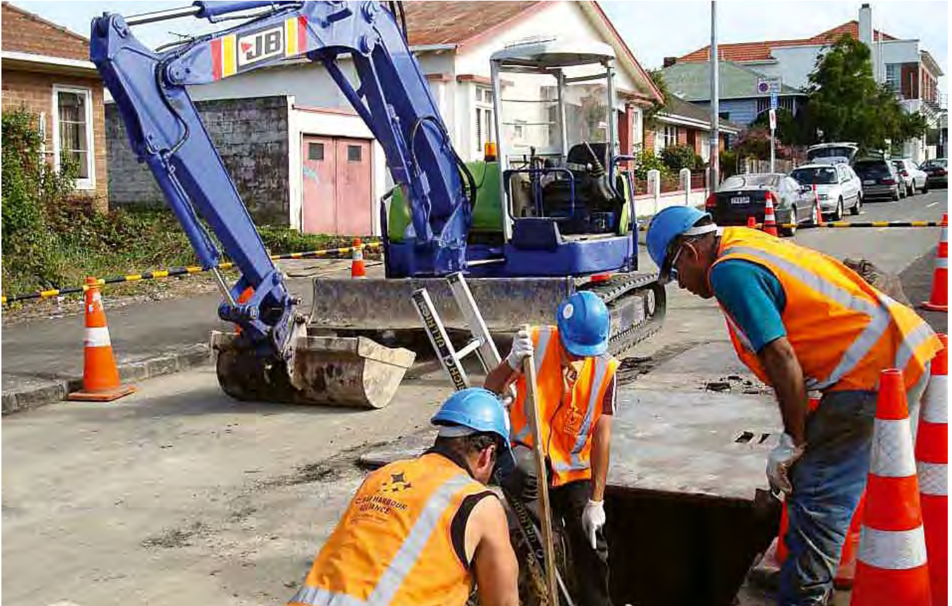
The project involved separating wastewater and stormwater pipe networks in densely populated areas of Auckland with many narrow and steep streets.
