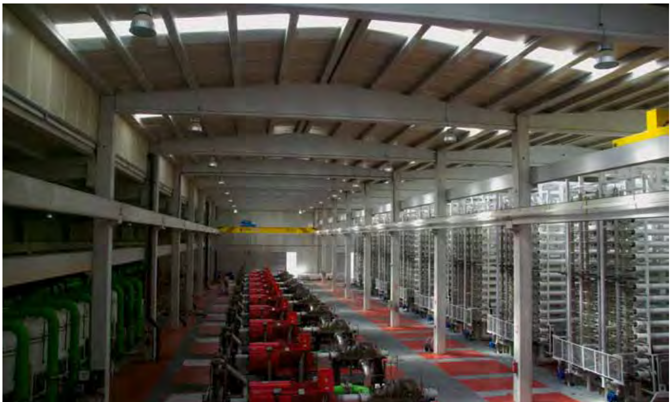
Inside the reverse osmosis building of Cartagena I. It is one of over 700 desalination plants in Spain that together provide more than 2GL/d of desalinated water for drinking and irrigation.
