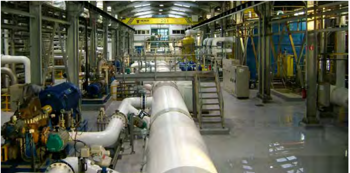
A 100ML/d seawater reverse osmosis desalination plant in Skikda, Algeria, was designed, built and is now operated by a consortium featuring Valoriza Agua. The plant supplies water to a population of around 500,000.
