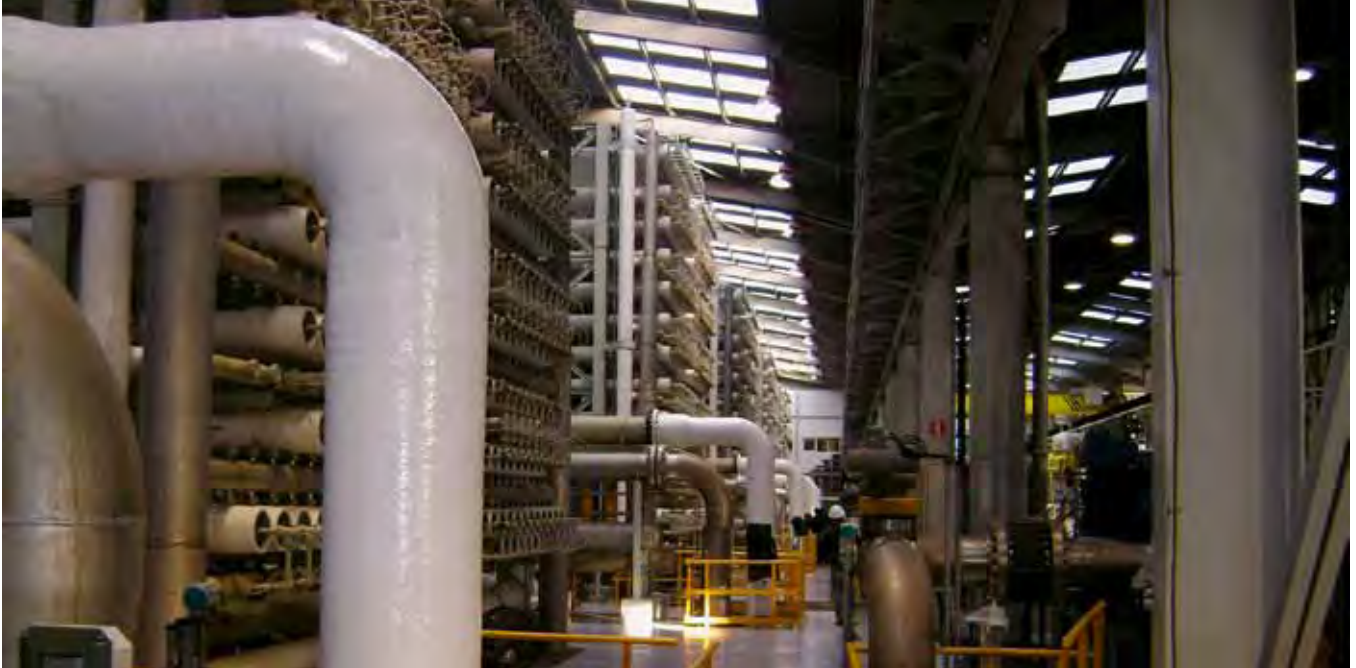
Abengoa companies Befesa and Codesa, ACS company Cobra-Tedagua and Sacyr Vallehermoso's Sadyt make up the Geida consortium, which was awarded the 25-year build-own-operate contract for the Skikda plant in April 2004.
