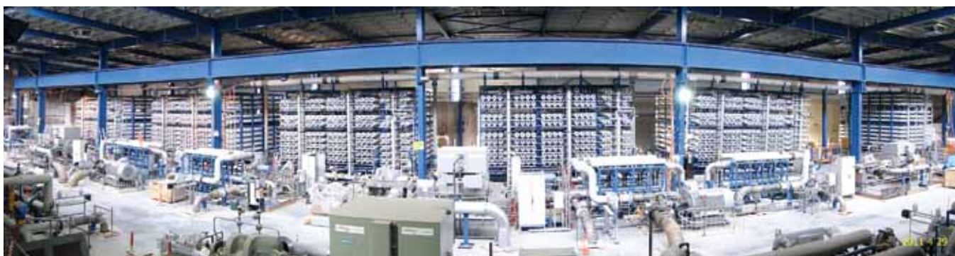
A view of reverse osmosis racks at the Adelaide Desalination Plant. The plant has 35,520 membranes in total.
